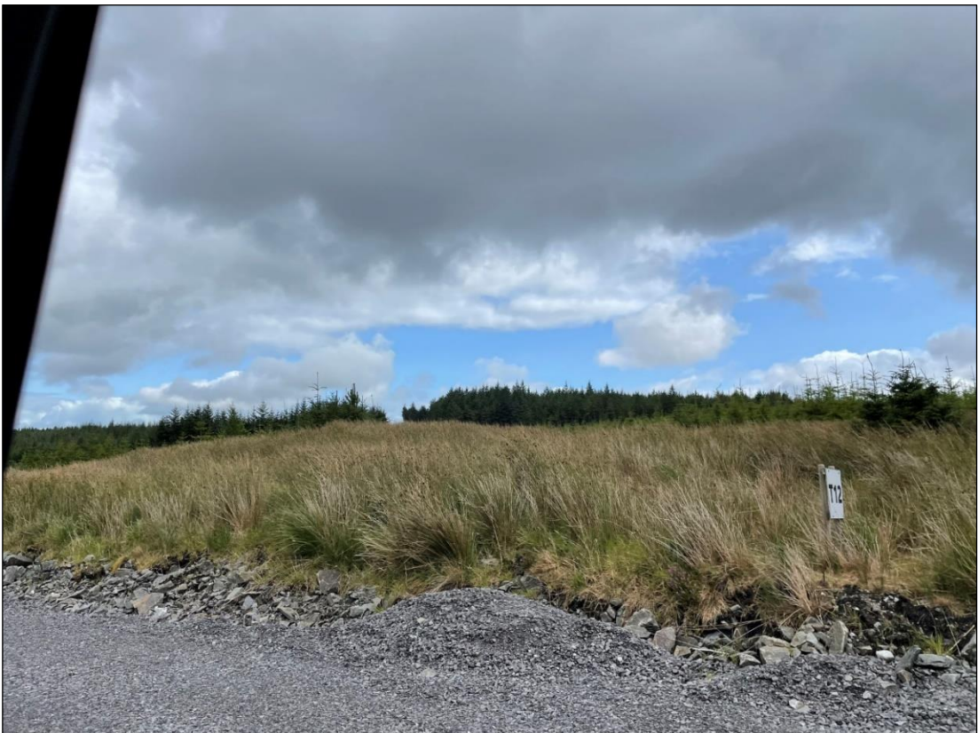
Plate 4--23 Site of minor deviation at Deviation 6 – road constructed approximately 30m downslope of the permitted to avoid excessive cut
